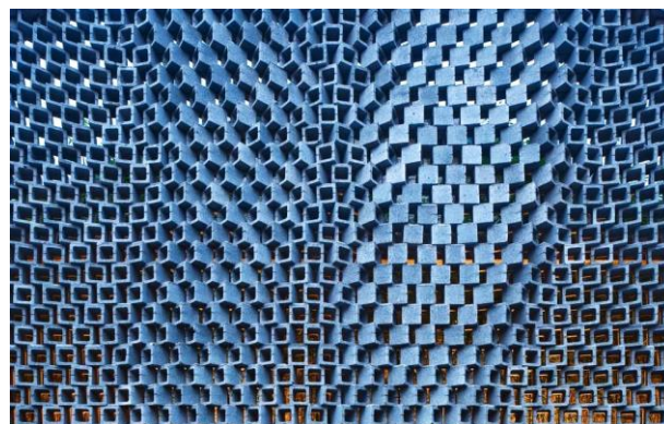
Fig.5 Yaw operation was done on the brick unit to allow light and shadows
