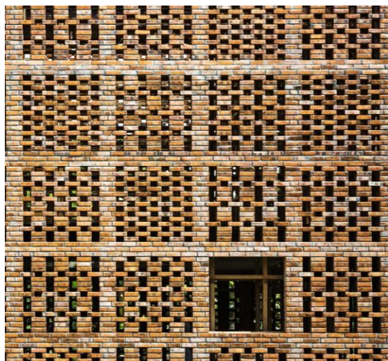
Fig.2 Selective and corbel operations were done to create the gap in the wall
