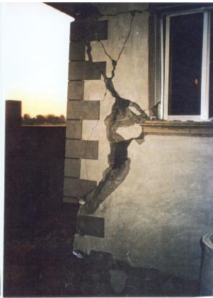
(b) Separation of wall at corner
