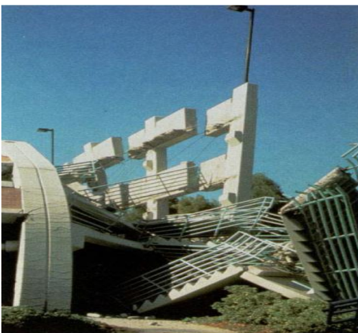
Figure 19 Collapse of parking garage
