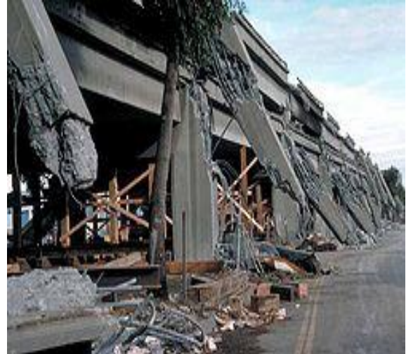
Figure 15 Collapse of expressway
