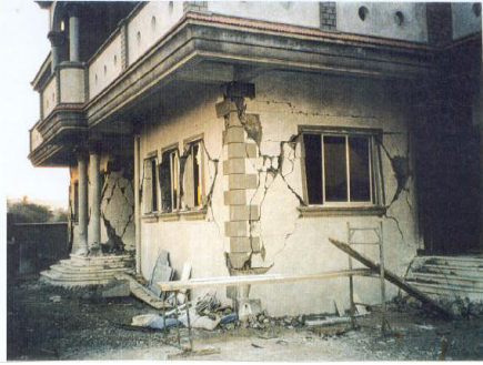
(a) Shear crack in wall
