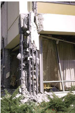
Figure 14 Collapse of concrete column
