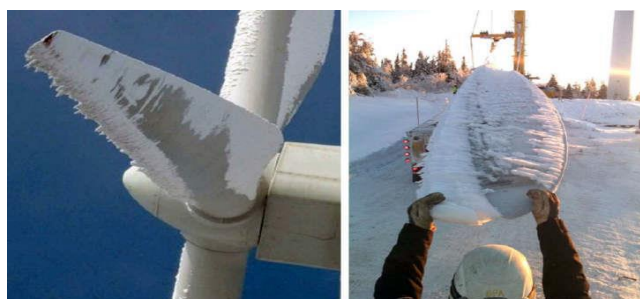
Figure5: Damaged Turbine Wind Blade due to Icing
