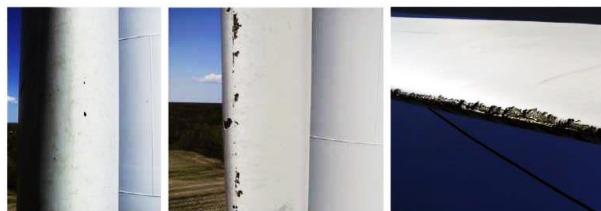
Figure 4: Damaged Turbine Wind Blade due to Edge Erosion
