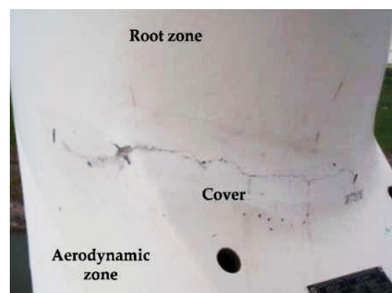
Figure 3: Damaged Turbine Wind Blade due to Fatigue
