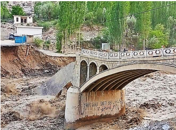
Figure 4 Hassanabad Bridge after Collapse
