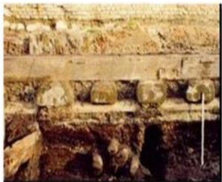
Fig 5: Typical view foundations historical building in Olsztyn, Gdańsk,(Ref. Przewlockia J., Zielinska M. (2016))
