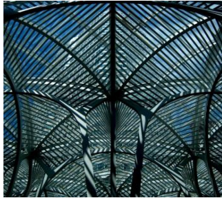
Fig.11 The engaging ceiling structure of the Allen Lambert Galleria and Atrium at Brookfield Place
