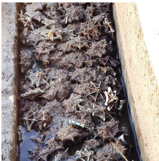
Fig.4 Accumulation of suspended solids over and inside the biofilter
